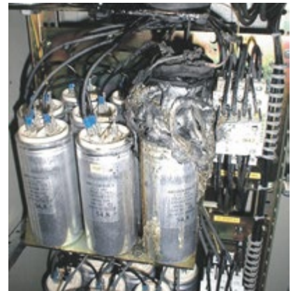
Fig. 6: Destroyed PP reactive power compensation capacitor: A creeping high-impedance ground fault has led to the complete melting of the capacitor and a localized fire.
