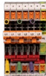
Fig.: Current transformer terminal strip
