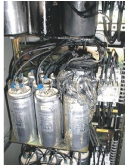
Fig.: Capacitors destroyed by harmonics current
